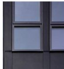
7 Painted fiber cement siding
